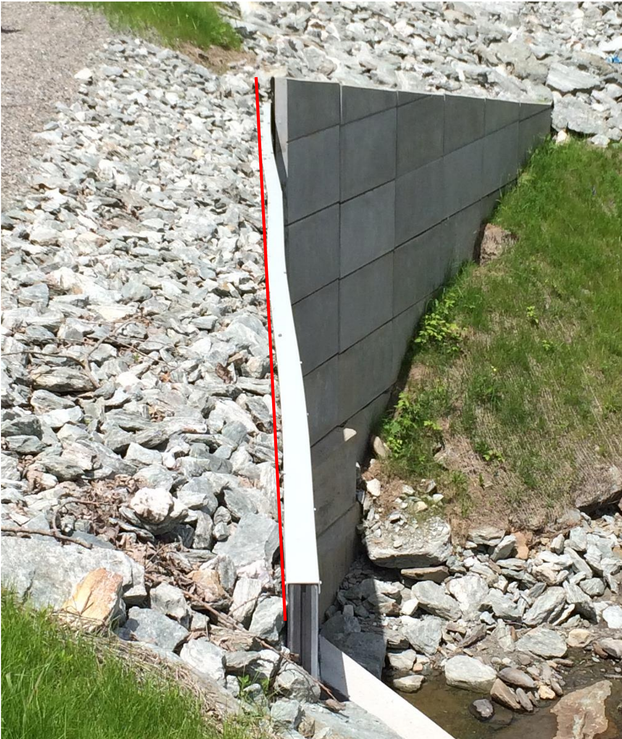
Figure 2 Easterly headwall bowing out with a meandering curved shape
