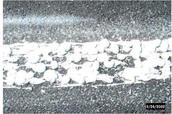
Figure 2. Initial installation – poor quality.
