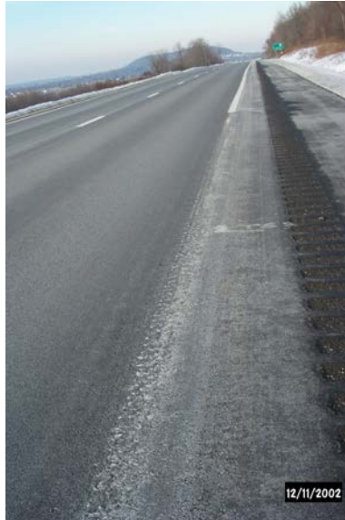
Figure 5. Drop-On-Line ® pavement marking system (foreground) after 2 ½ months of service vs. standard thermoplastic (background).
