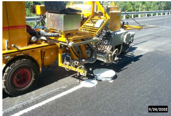
Figure 3. Equipment problems – operations halted.
