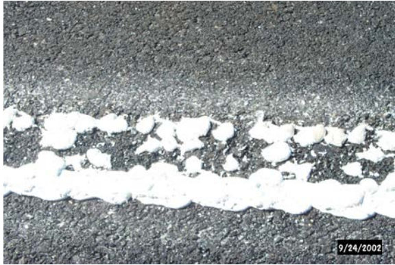
Figure 1. Initial installation – poor quality.
