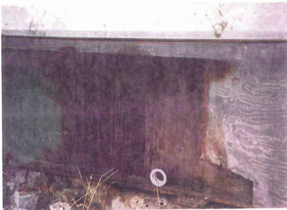
Rusting at end of Beam.
