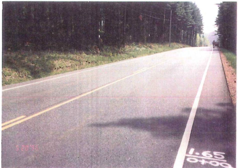
No distress noted in treated lane (east-bound) or untreated lane (west-bound) at MM 1.65
