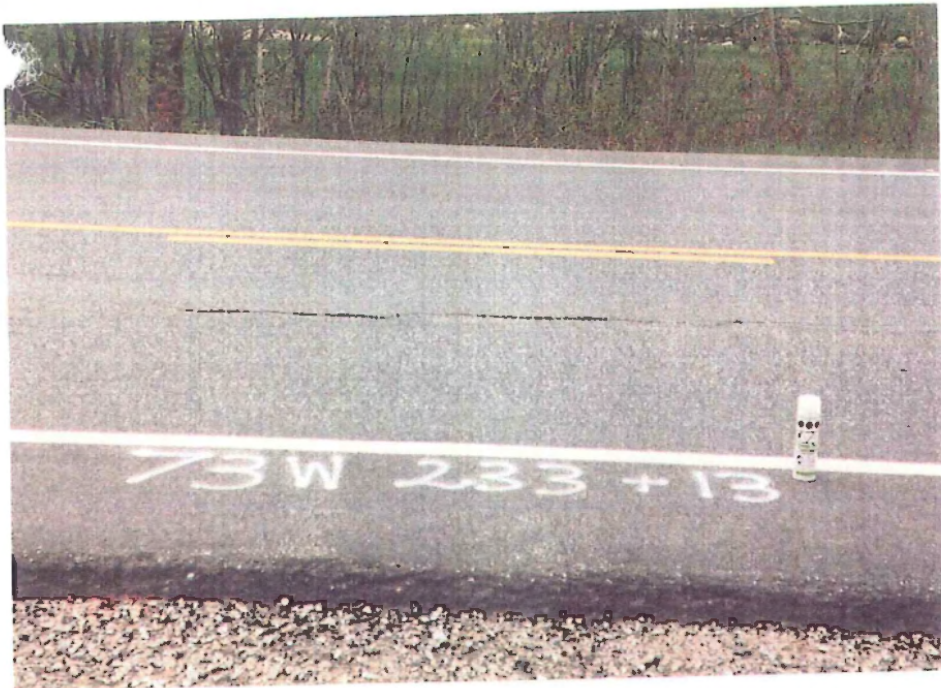
Longitudinal cracking in untreated test site at MM 2.33
