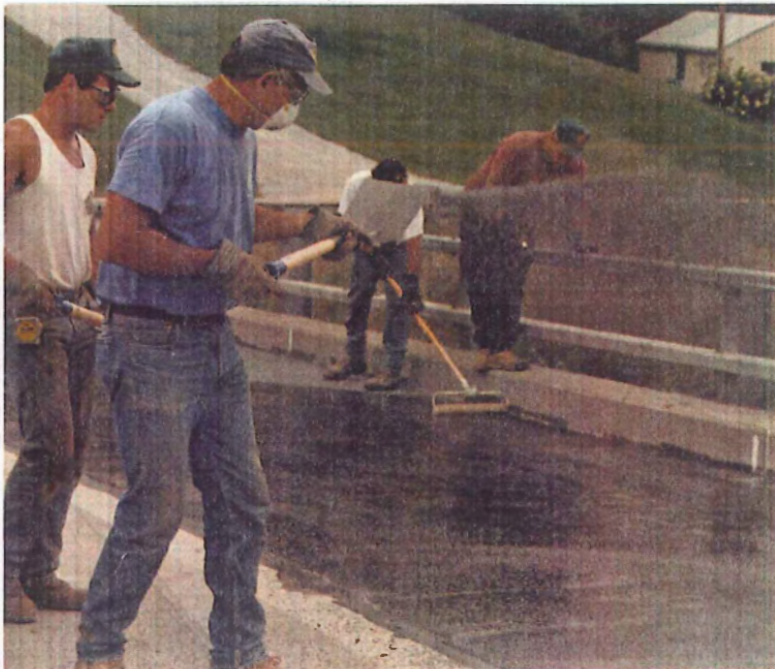
Thin polymer overlay is applied with rollers while basalt aggregate is broadcast over the surface.
