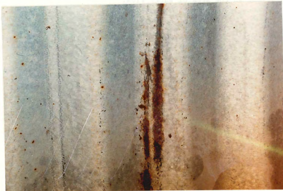
Note band of corrosion plus random spot corrosion
