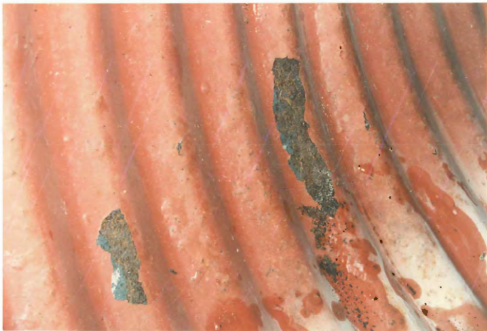
Note blisters in coating and complete corrosion where the epoxy was removed for inspection
