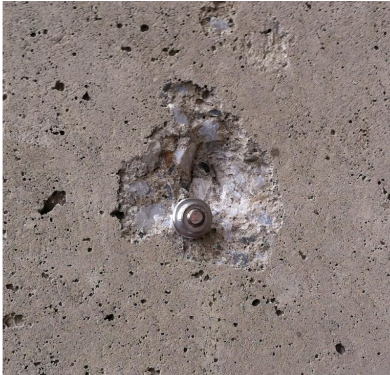
Figure 3 Powder Actuated Faster Caused Concrete to Burst.
