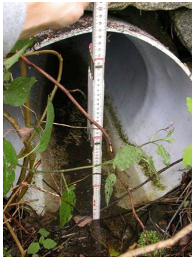
Figure 6: 18-inch pipe outlet, 2007
