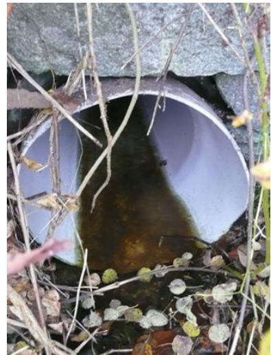
Figure 7: 18-inch pipe outlet, 2010
