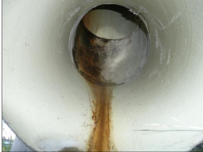
Figure 4 - Iron Oxide Discoloration 2010
