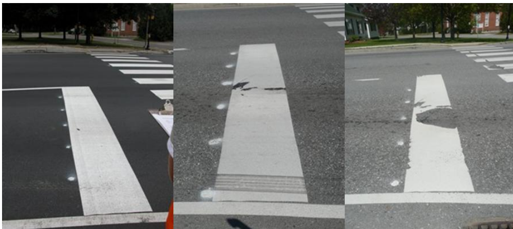
Figure 4. Progressive wear characteristics of test site 3, from left to right, at 0, 8, and 19 months post construction.
