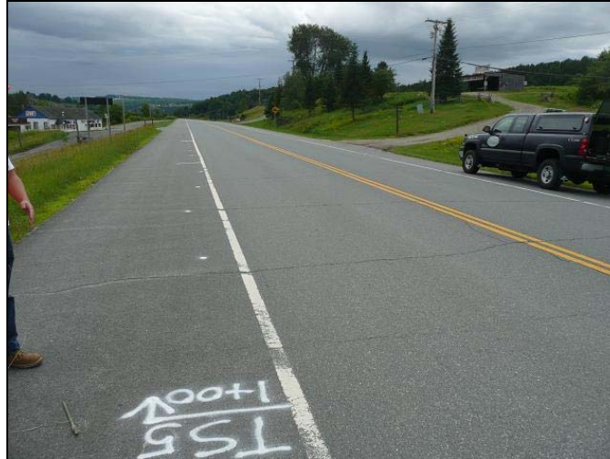
Figure 7. Typical Thermal Cracking
