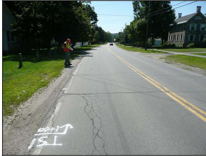
Figure 4. Typical Fatigue Cracking
