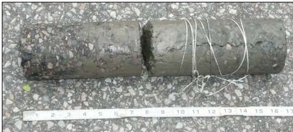
Figure 6 Core Extracted Over Crack
