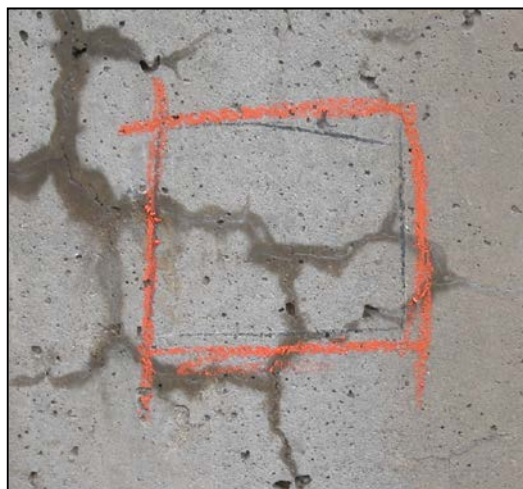
Figure 1 Crack with white precipitate.
