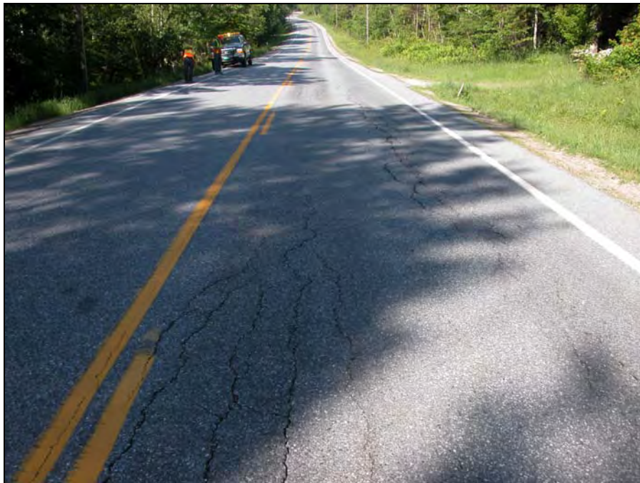
Figure 2 – Typical Fatigue Cracking
