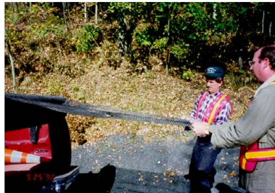
Figure 6 – Installation in Barnet
