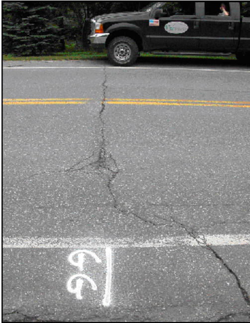
Figure 11–Crack 24m south of edge, 2007
