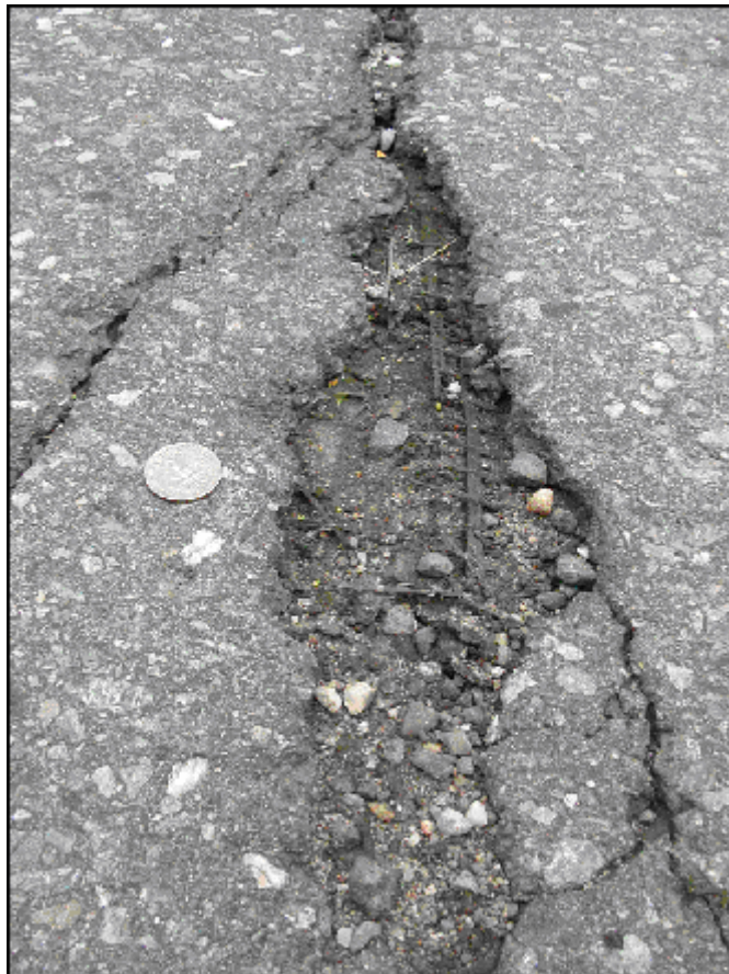
Figure 13 - Exposed GlasGrid material, 2007
