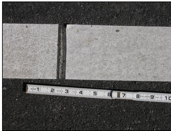
Figure 2 – Void Between Tape Segments
