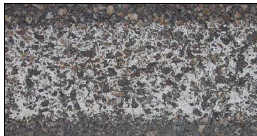
Figure 6 – Test Site 5 White Edge Line May 30, 2007, Wear Rating = 4
