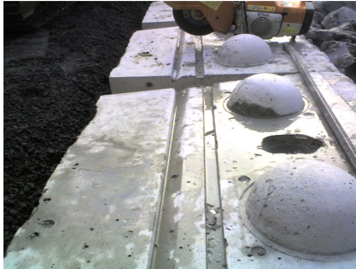
Figure 8: Reinforcing steel channels out of alignment
