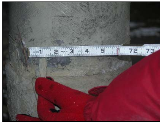
Figure 3 – Flaking of Adhesive
