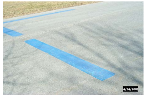
Figure 12. Test Strip B after eight months.
