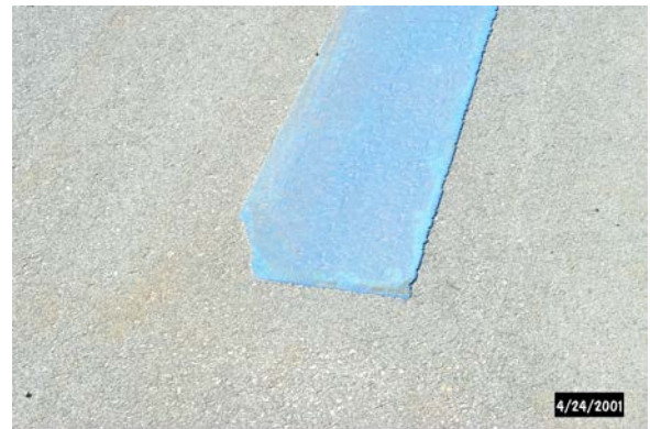
Figure 14. Test Strip B (west end) without feathered edge after eight months.
