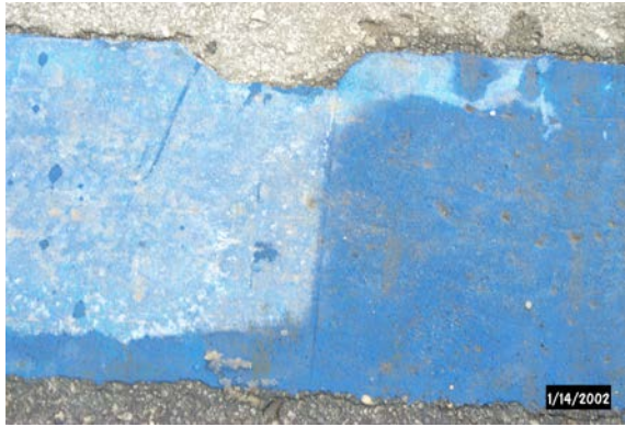
Figure 18. Detail of plow damage after 17 months of service.
