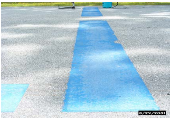
Figure 16. Test Strips A and B after 12 months of service.
