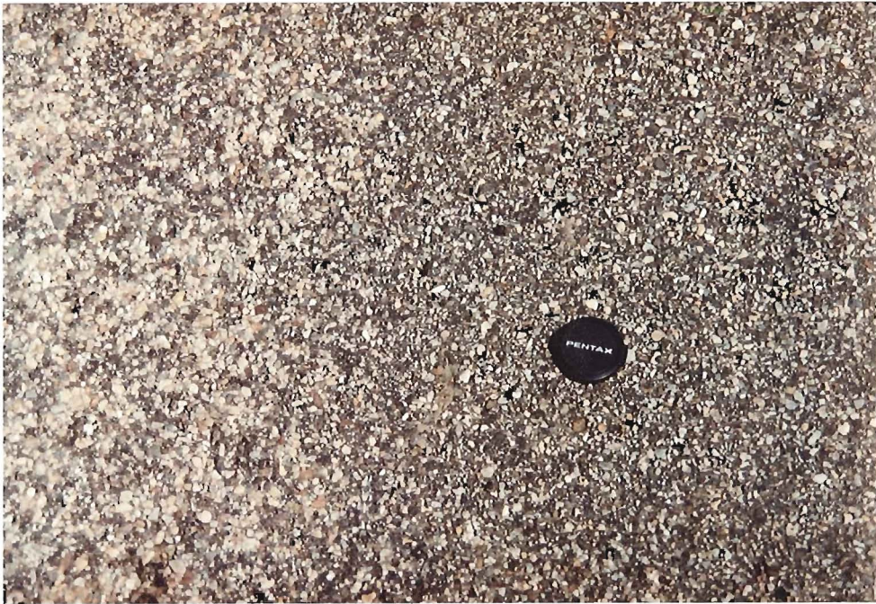
Condition of Surface Treatment
