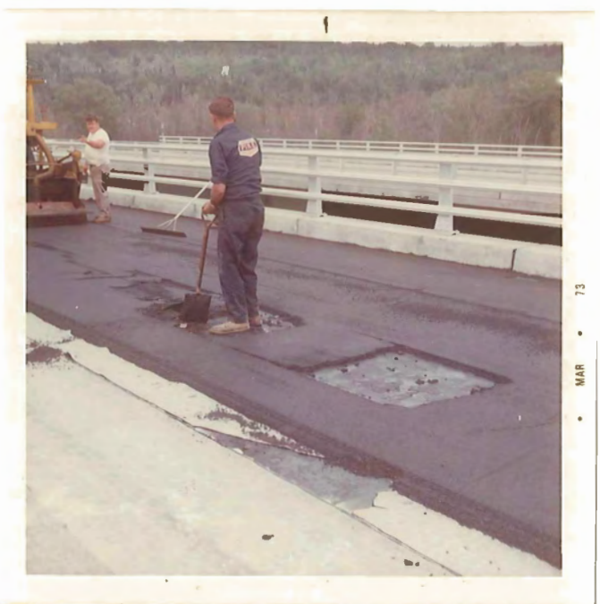
Lack of bond between roofing sheet and polyurethane caused blockage of the paver screed
