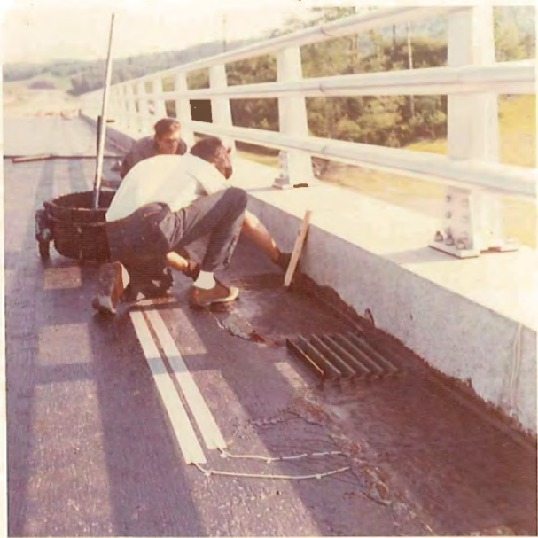
Copper foil strips placed beneath a membrane to detect the passage of moisture
