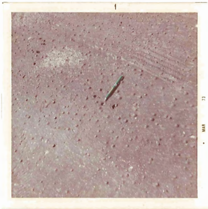
Visual checks of air bubbles in a hot applied rubberized asphalt disclosed that most were open to the concrete
