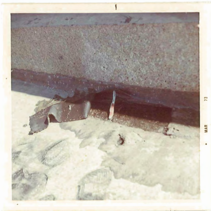
Water detected beneath top course of rubberized asphalt and rubber sheet along the base of the granite curb
