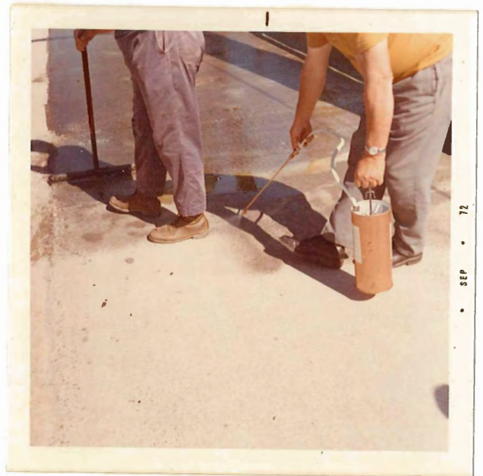
Applying first coat of the clear epoxy. Note the spray application of water
