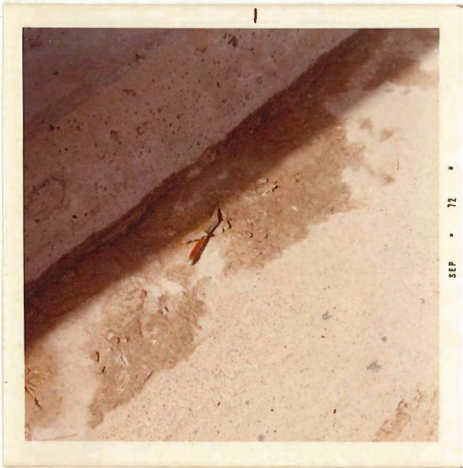
Laitance along westerly curb
