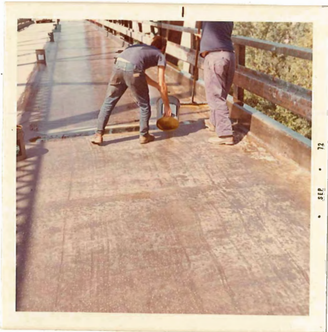
Applying second coat. Note dry looking areas where the first coat of epoxy appears to have penetrated into the concrete
