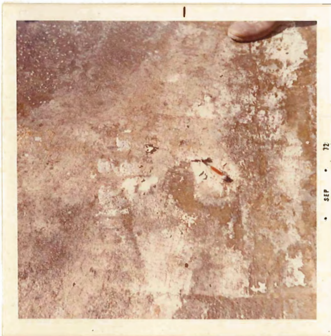
Inspection of first coat of epoxy revealed that the material had not penetrated into areas of heavy laitance
